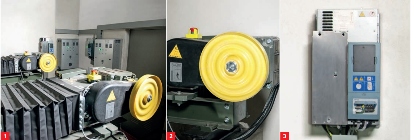
1: Set-up in machine room | 2: Hand wheel for manual rescue | 3: Frequency regulation
